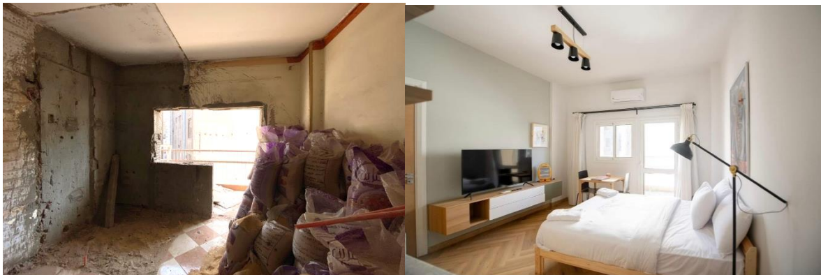
Figure 18. The photos above demonstrate the before and after status of one of the studios in the project.
