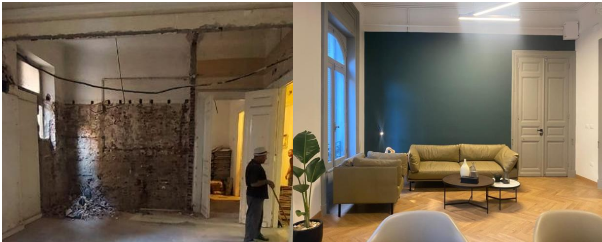
Figure 11. Before and after photos of what currently is a meeting room; the previous tenant destroyed the original window and created a wall in its place. Transgressions were removed and a new window replicating the original design was added once again.
