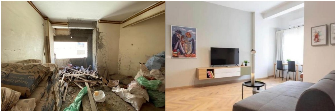
Figure 16. Before and after photos showing how the openings and windows were restored to their original size and look to maintain the harmony of the building's façade.
