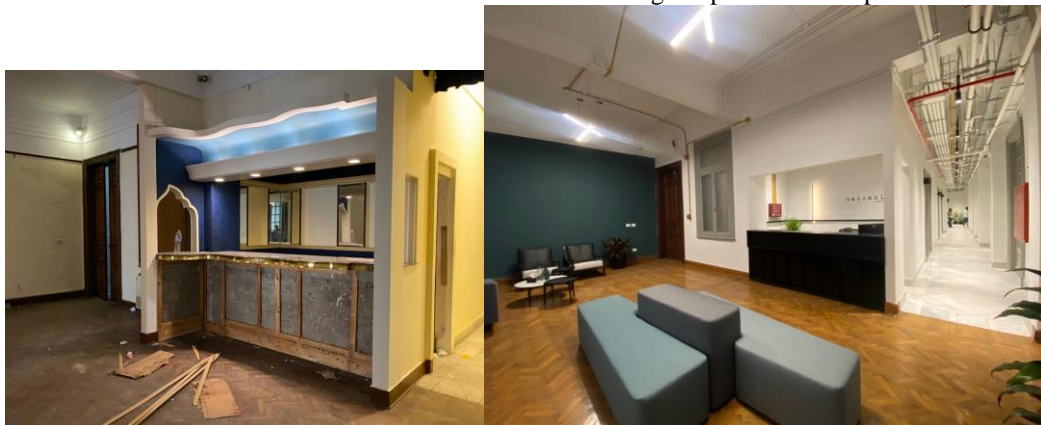
Figure 9. Before and after status of the reception area of the project, the original parquet floors were restored and the existing features were maintained. Electrical systems were installed in an exposed manner in order to preserve the vast heights of the interior spaces.
