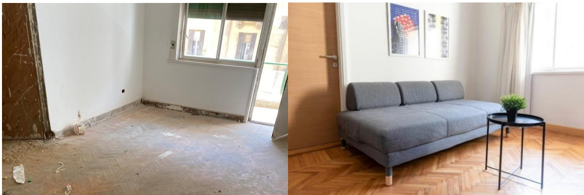
Figure 17. Before and after status of one of the units which had original parquet floors, those were restored and reutilized in the space, also another feature that was restored was the original windows and roller shutters.
